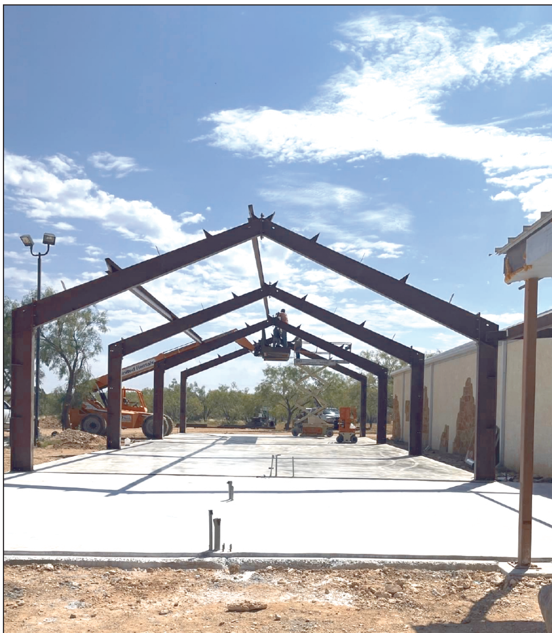
Construction Zone! Work continues on the new exhibit space and theater at Fort Chadbourne.
