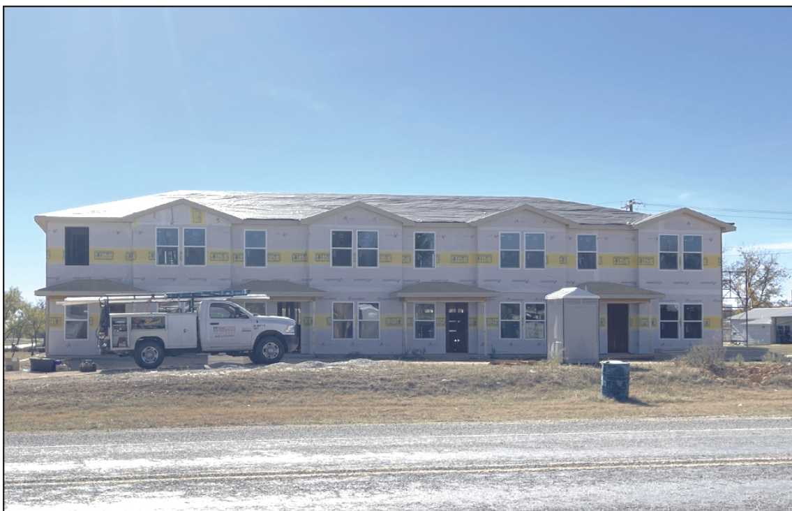
Changes! Construction continues on the housing project near the water tower in Bronte on the afternoon of Monday, December 11.
